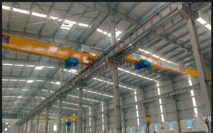
Multiple EOT Cranes
