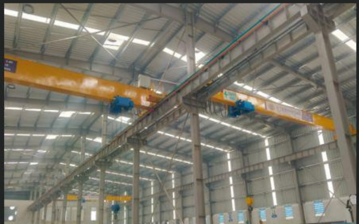
Multiple EOT Cranes
